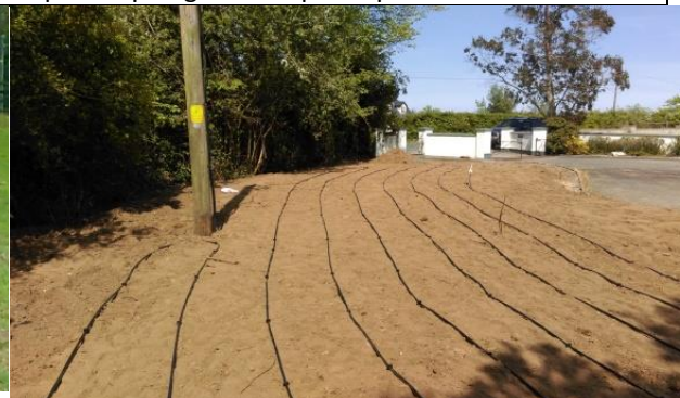
In shallow soils sand is added below the driplines to increase soil depth, with the dripline pegged on the exposed area and backfilled with 200mm topsoil.
