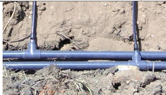
Driplines are connected to PVC pump supply and return manifolds via the headworks
