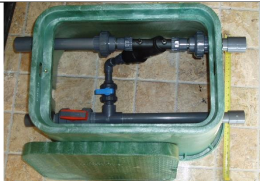
Pre-assembled headworks with filter and valves
